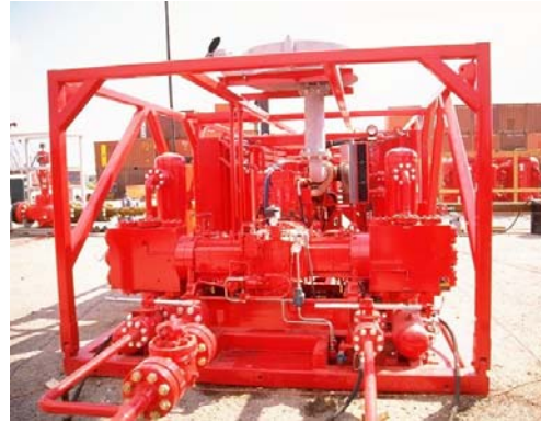
Figure 3: High pressure booster
