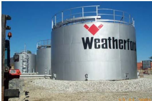
Figure 4: Fuel storage tank
