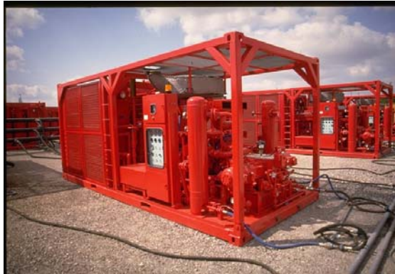
Figure 2: Main compressor unit
